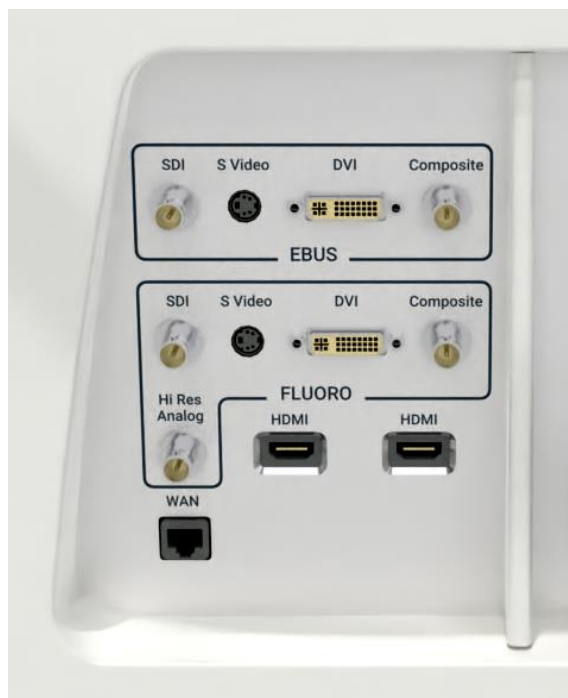
Figure 5.2 Audio Visual (AV) Connection Panel
